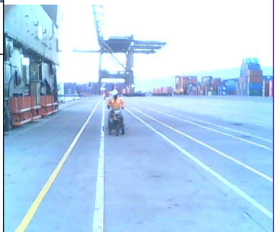
Andre Beckford line striping the terminal apron. This is a tedious process involving a high level of accuracy.
